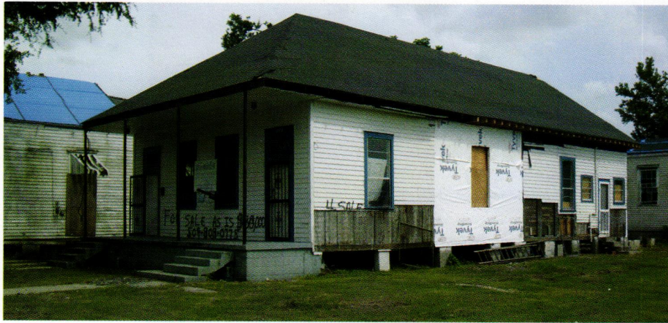
The house on Dauphine Street is in the process of being restored thanks to PRC, the Traditional Building Exhibition and Conference, architect David Dillard, and the projects many sponsors who donated materials.
