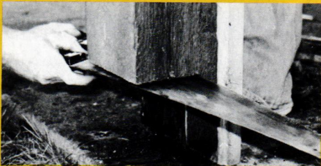
10" rotted bottoms of these load-bearing columns...
