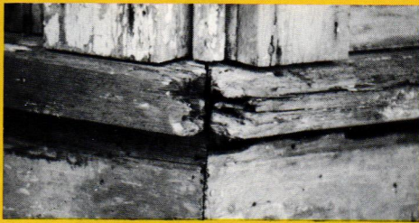
This rotted – and irreplaceable – woodwork...
