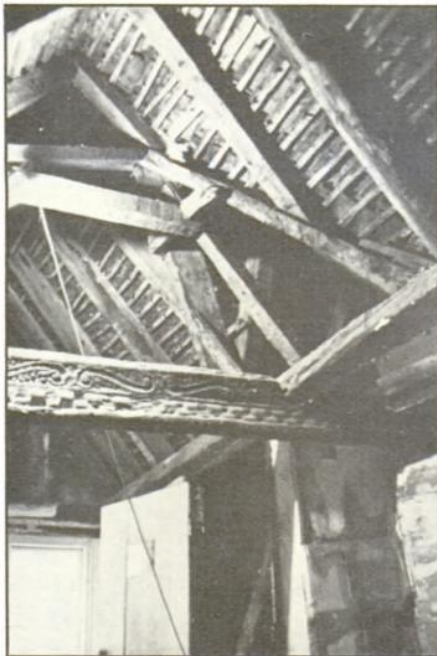
The attic room showing how the timbers are joined. On the right side is a bit of "wagenschot" and across the middle is the carved cornice.
