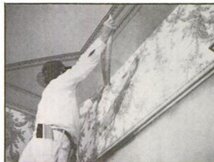
After the vertical panels are on, Albert Moll applies the border and frieze strips to the wall to complete the wide border effect.
