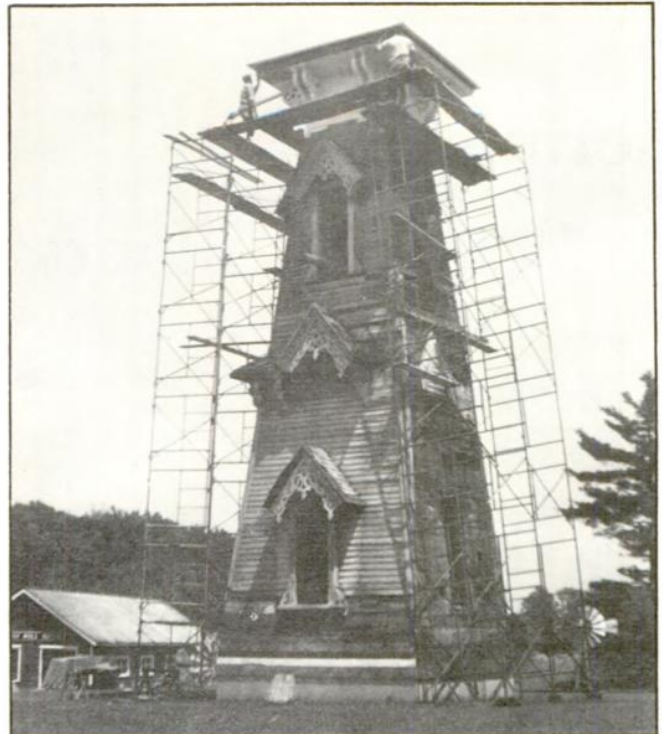
The extensive repairs necessary for the gingerbread, clapboards, etc., required full scaffolding to be set up.
