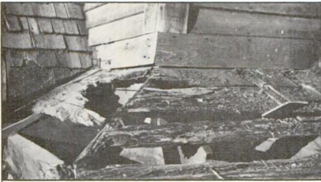
This section of the mid-tower roof shows the extent of deterioration.
