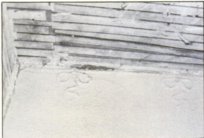
Two plaster bow ribbons on the second floor wall were all that remained of the original decorations.
