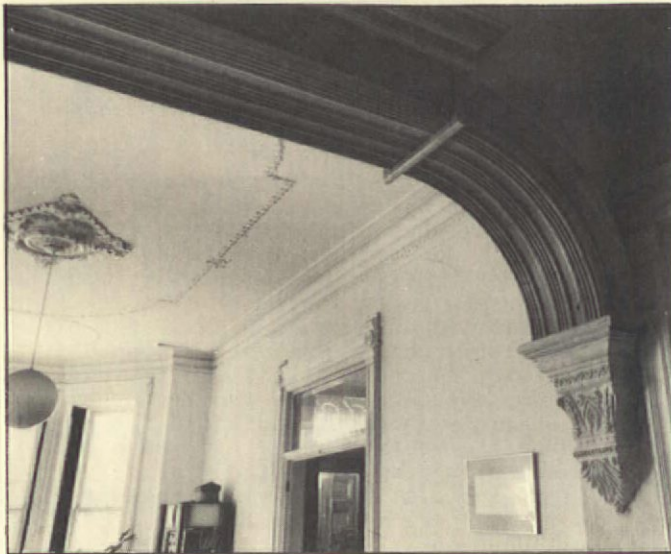
Evidence pointed to a plasterwork arch between the front and back parlors. Bill reconstructed the arch in wood with plaster corbels.
