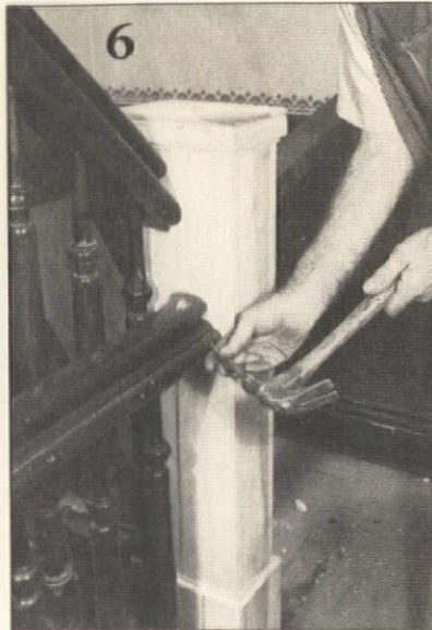
Countersunk nails hold the rails to the newel. Had this been a fine parlor stair, Harry would have taken the trouble to install a hidden rail bolt. (see OHJ, June 1981, p. 138)
