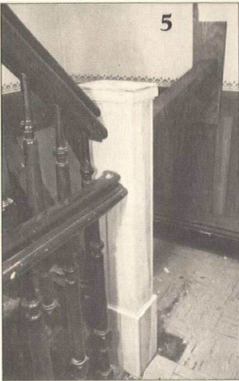
The newly-installed replacement newel is temporarily braced in a true vertical position, awaiting nailing. It will be nailed into the floor, the bottom step, and to the handrails.
