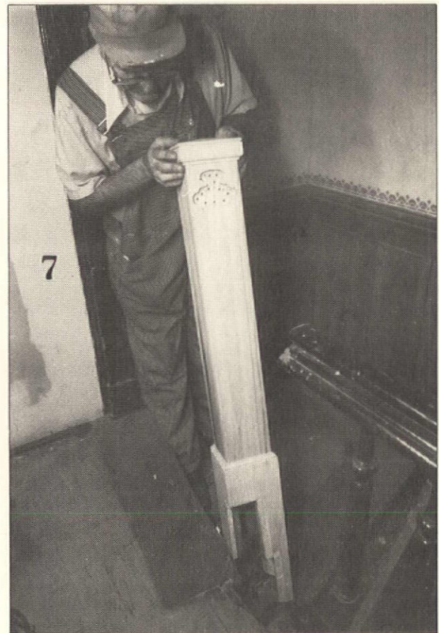
Harry installs the second replacement newel. (Marks in mirror are from a drill bit used to rout out most of the wood.)
