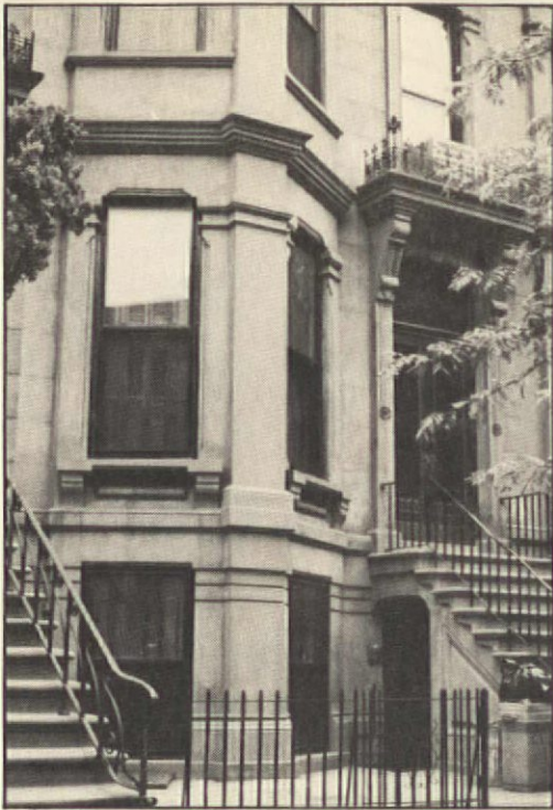
Both of these previously unpainted brownstone buildings were spalling. Their owners hired contractors to do color-matched patches, so the headache of periodic maintenance painting could be avoided. Left: The contractor who worked on this job had an ex-
