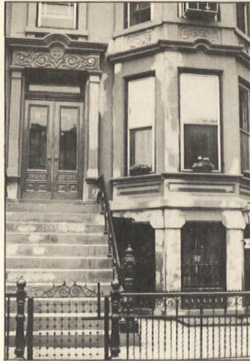
cellent reputation. Right: This contractor had a spottier track record (pardon the pun), and the owner didn't insist on a test patch. Now it's either regular painting or permanent scars.
