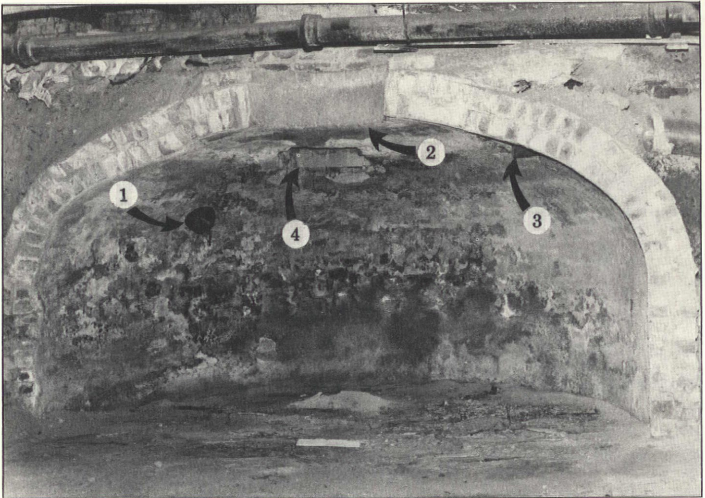
This extremely rare cross-section view of an in-ground cistern was taken by subscriber Craig Wolf. The cistern, built c. 1876 in Beacon, N.Y., was originally located a few feet from the house. However, an addition to the house resulted in the cistern being half inside the new
