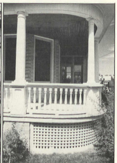
The verandah on this house in Logan, Utah, shows how lattice could be curved to suit the building's requirements. Wood screws were used at the lattice intersections to join the front layer with the back one.
