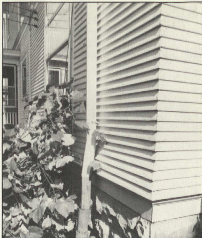
The gutter downspout appears to be feeding into a house sewer connection, but the clay tile elbow is actually one of two inlets for the basement cistern. When the cistern was first reactivated, leaves washed down into the cistern and caused an odor as they decayed. Putting a nylon net strainer over the downspout where it enters the tile elbow solved the problem.
