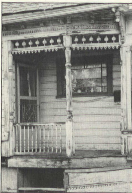
Severe structural problems, not to mention the missing lattice work, had befallen the Best/Cannon House prior to its rehabilitation. Note the newly installed concrete foundation that replaced a collapsing brick one.
