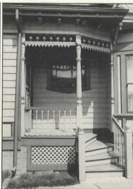
Here is the same porch after rehabilitation; the new lattice is installed back in its original position below porch and steps. Note how the concrete foundation has been clad with brick to resemble its original appearance.
