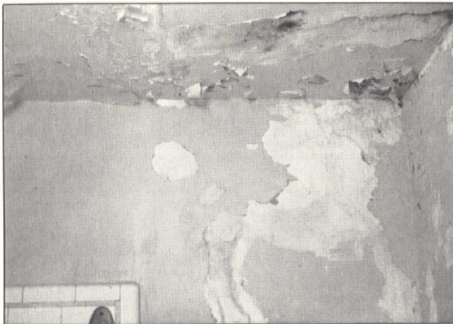
The best way to rescue a wall such as this one, with its water-damaged plaster and peeling paint, is by applying lining material.
