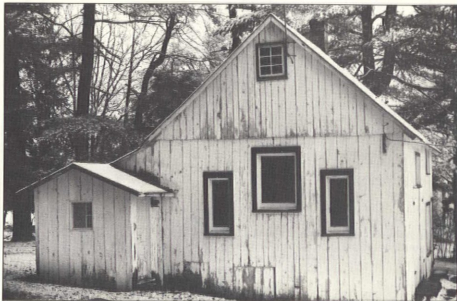
Neglected whitewash -- an outbuilding on the author's property.
