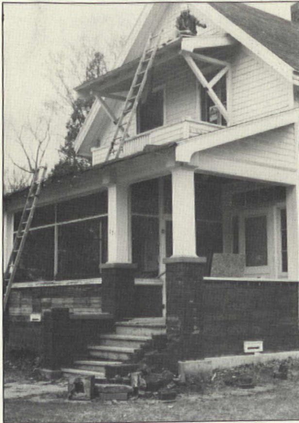
Restoration of the original Greek Revival facade began with the demolition of the pseudo-bungalow porch and awning.
