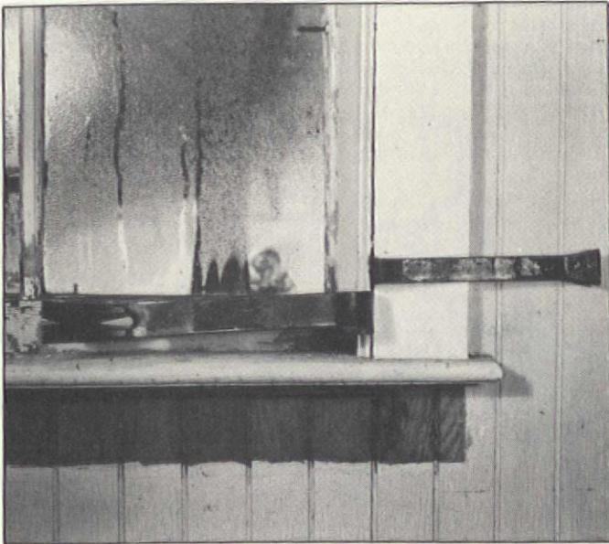
Using two prybars in opposite directions is the easiest way to remove the stop moulding of a window.
