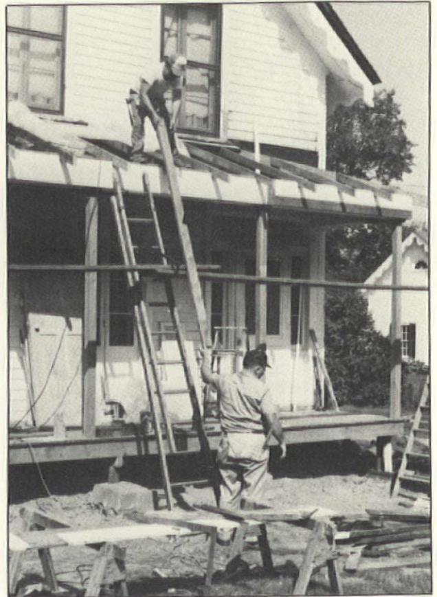
Half-way through the restoration. The Crosses duplicated a piece of the original bargeboard that they found under the eaves.
