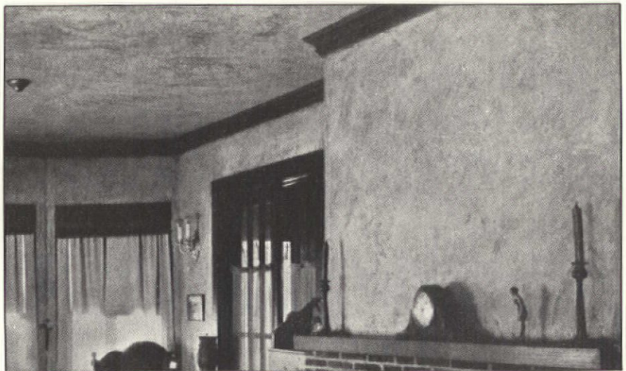
The walls and ceiling of this room have been finished with a Holland plaster wall texture, a finish which is shown in detail in Illus. 1 on the next page.
