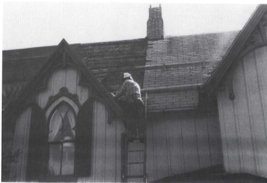
Rick is flashing a dormer valley in preparation for the new shingles. (Weren't the old shingles attractive?!)
