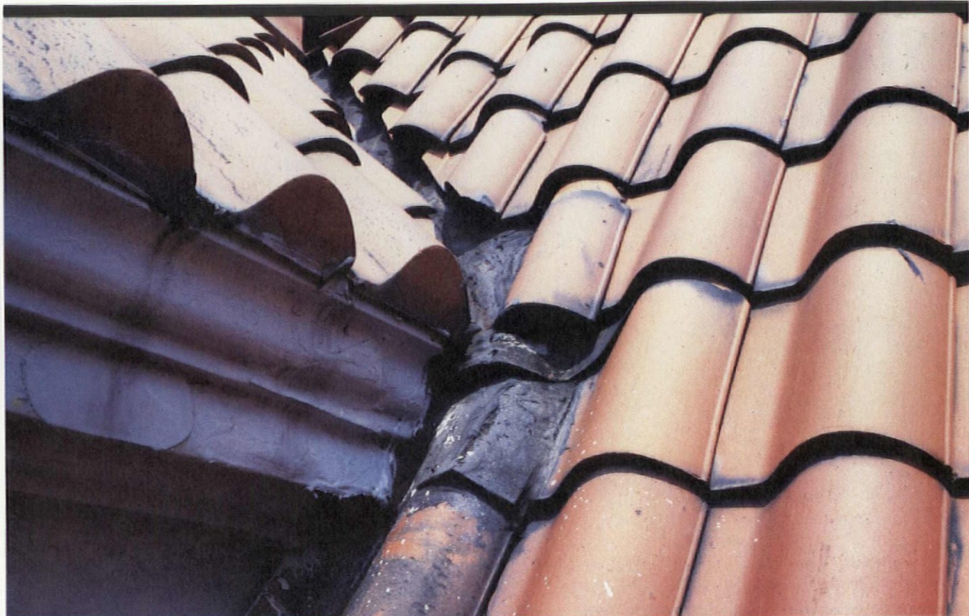
Asphaltic "goop" was sloped on eroded flashing, accelerating corrosion of the metal cornice.
