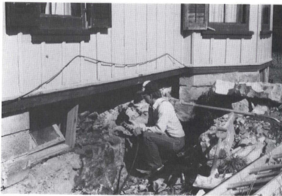
These photos show that our house was restored top to bottom. What good is a new roof without a solid foundation?
