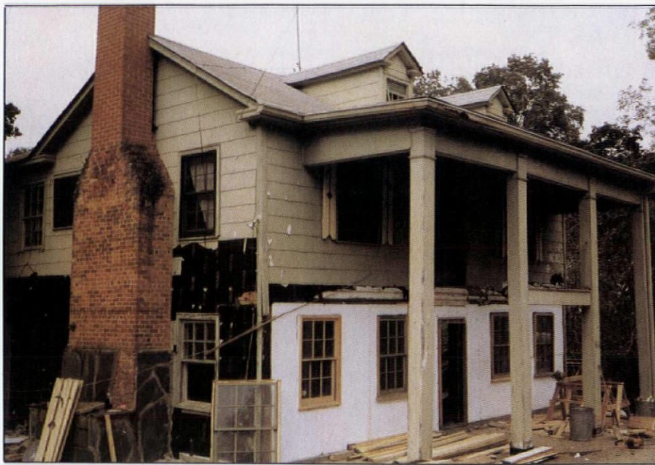
A major project was removing the asbestos shingles which had been placed on the house sometime during the late 1940s or early '50s.
