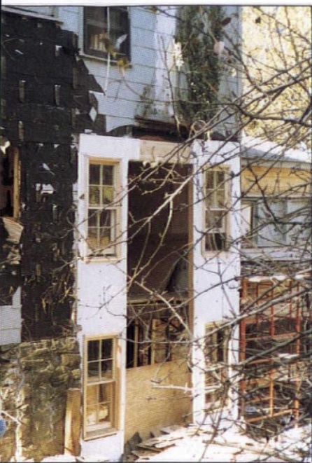
What happened during the restoration the siplap was for the most part unusable.
