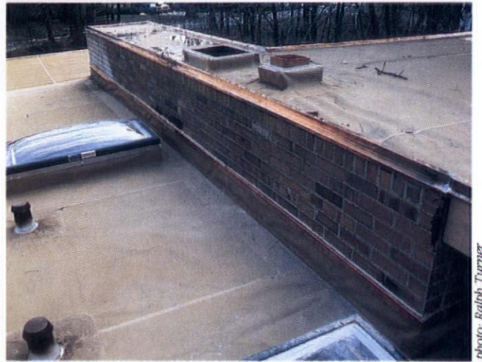
Above: a view of how the membrane is treated around the chimney flue as well as the copper cant and chimney flashing.
