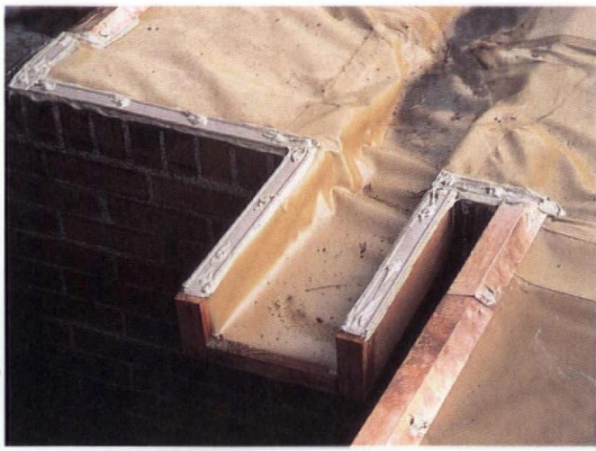
Water near the front doors was eliminated by taking the built-in drain over the brick wall and ending it at a scupper. Water spills into a gravel crock below, filled with 2" stone, Japanese-Great Lakes in appearance.
