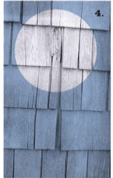
Sapwood decay has eroded enough of this shingle to expose the nail in the course below it.
