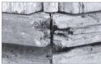
This rotted - and irreplaceable - woodwork...
