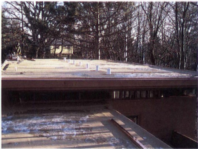
A roof, flat or otherwise, must breathe in order to last. The Duralast system includes venting boots to keep moisture from the bottom of the membrane. We used them to straddle each framing interval at the rafter, venting two joist spaces at the same time.
