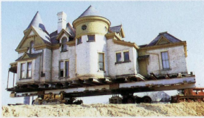
Technically, no house is too big to move. The real constraints are often time and money.
