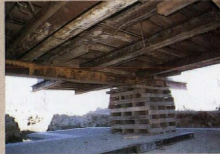
Once off the foundation, the building sits on a network of steel beams.
