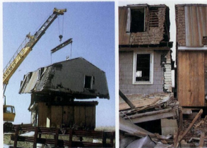
The Cook House had to be sectioned in order to make its 125-mile journey practical. Left: removing the roof by crane. Right: cutting away the added wing.
