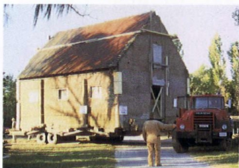
The solid-brick stable moving off the old foundation and onto the road.
