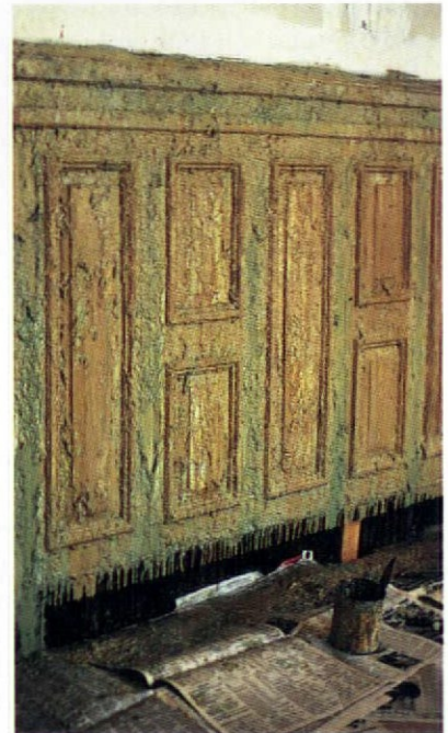
Semi-paste strippers contain thickeners to keep them on vertical surfaces. Drop-cloths and masking are still necessary to protect other areas and collect drips and scrapings.
