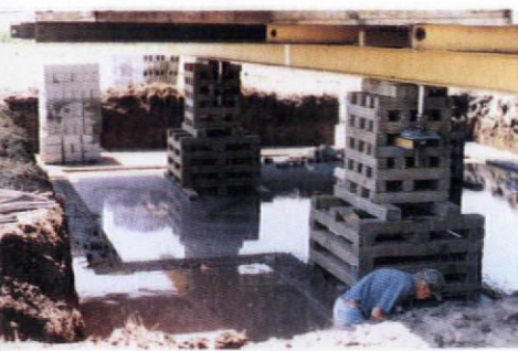
Footings may be pre-poured, but most foundations are built up to the house.
