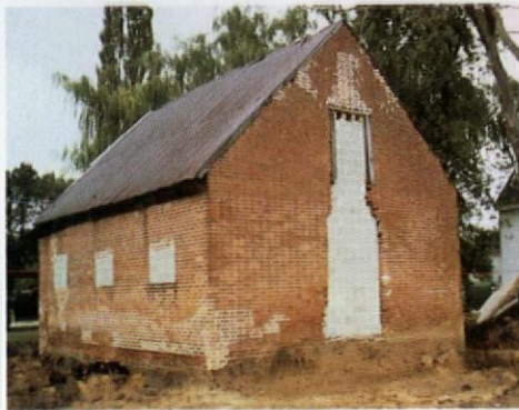
Preparing the stable by blocking in wall voids and excavating the foundation.
