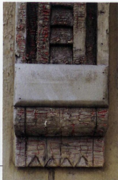
Far left: Peeling down to bare wood may be caused by water-vapor migration. Left: Poor preparation can lead to peeling between coats.
