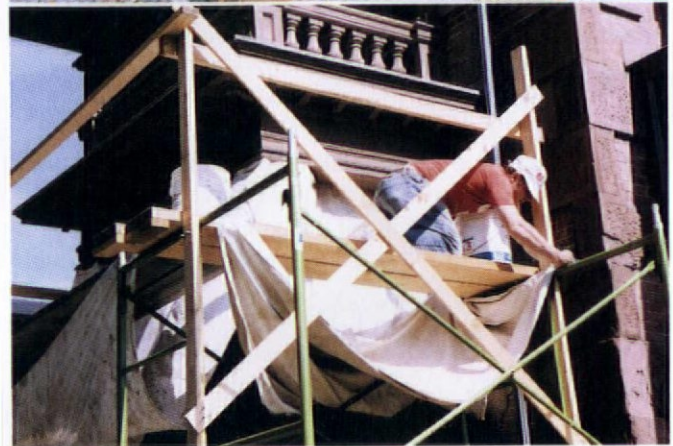
Top: Anne-Marie Lord prepares a wood balustrade by stripping heavy sanded-paint buildup with steel scrapers (which must be resharpened frequently) and a chemical remover. Above: Safe, stable scaffolding allows the team to concentrate on the sanded paint. Tarps control drying and overspray.
