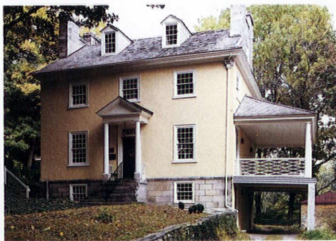
The Federal-style, stone and stucco house in 1990, after being repainted with acrylic latex paint.
