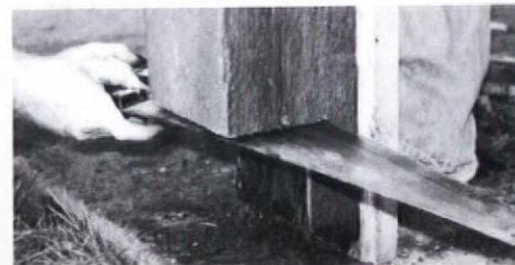
10" rotted bottoms of these load-bearing columns...
