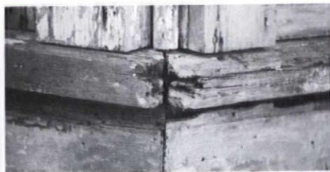
This rotted - and irreplaceable - woodwork...
