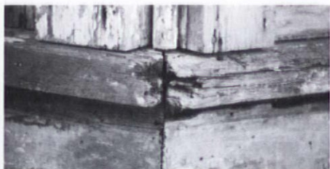
This rotted – and irreplaceable – woodwork...
