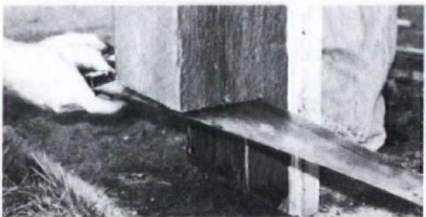
10" rotted bottoms of these load-bearing columns...
