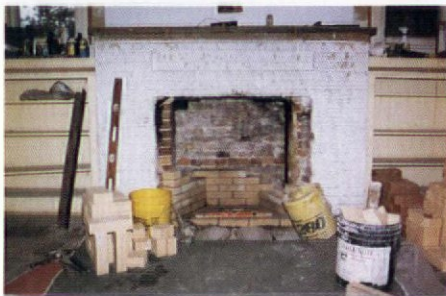
Top: A good work area has raw materials and soaking brick right at hand. Bottom: Laying in new firebrick.
