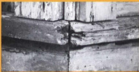
This rotted – and irreplaceable – woodwork...
