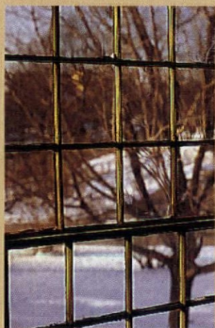
Divided light windows, in all their various configurations, are classic old-house details that can be repaired instead of replaced.
