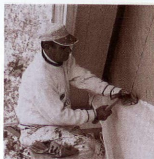
When the paint fails, installing new canvas and rosin paper is the only solution.
