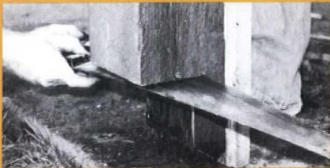
10" rotted bottoms of these load-bearing columns...
