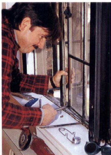
Steel window restoration expert John Seekircher straightens a warped vent at the author's home.
