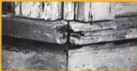
This rotted – and irreplaceable – woodwork...
