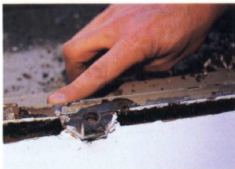
Weep holes should be opened up so that water can drain to the exterior.
