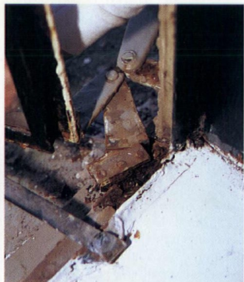
As the vents are being aligned, the contractor should check the hinges. They may have rusted and come loose from frames or vents.
