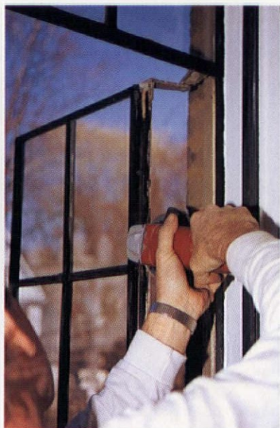
Far Left: Use an angle grinder with a carbide disk blade to remove built up paint and rust. Left: Clean window pockets and edges of vents so the window closes properly.
