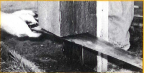
10" rotted bottoms of these load-bearing columns...
