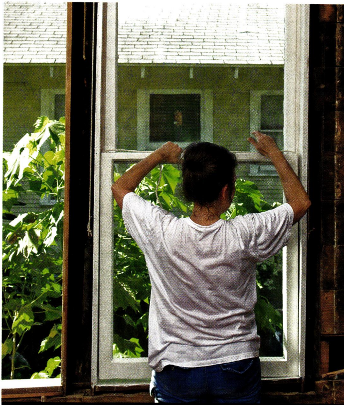
After replacing the top sash and tying on and adjusting the weights, Pam fits the bottom sash into the window.
