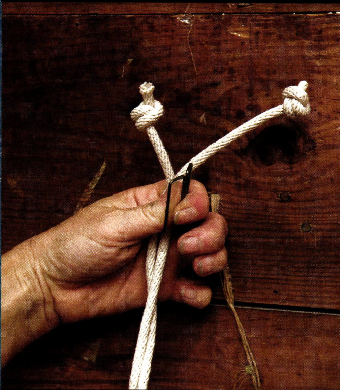
To attach sash rope securely, Pam prefers to use staples ("my insurance package," she says) in addition to nails.
