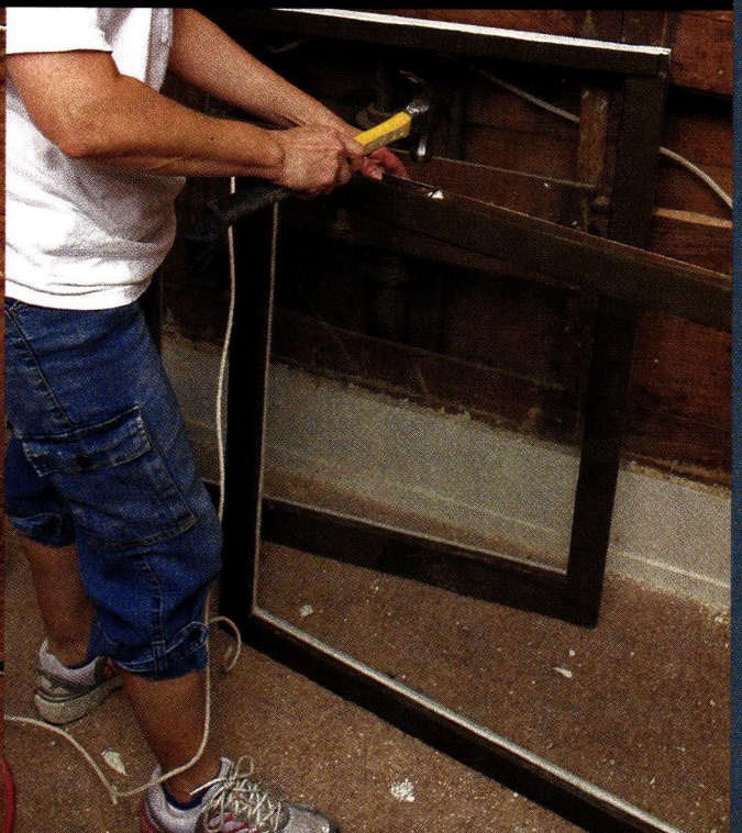
Pam nestles sash rope into an existing hole, then hammers it in place. The length of the rope fits into a routed channel along the sash.
