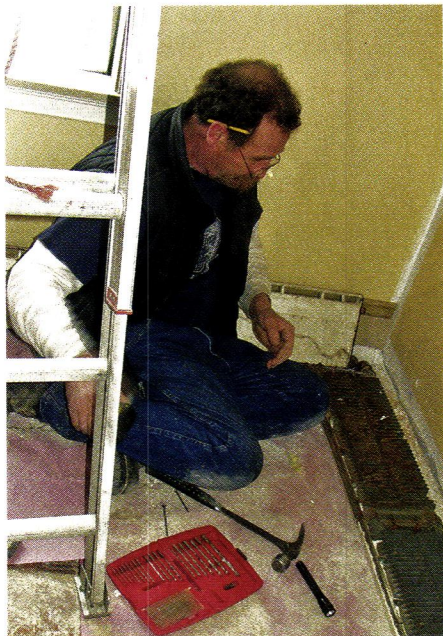
Inside the tower, tight space proved challenging for the work team to negotiate.
