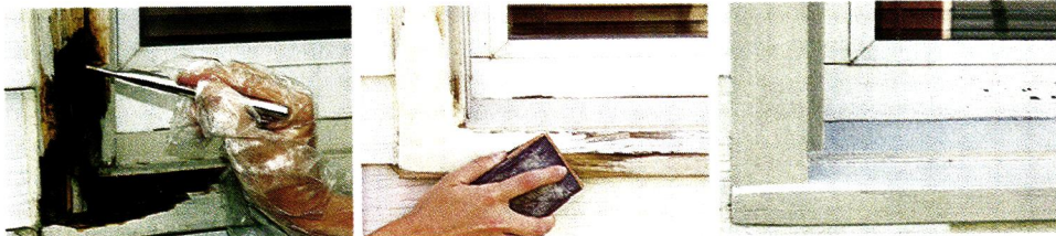
Restoration of rotted window is easy and cost-effective.
