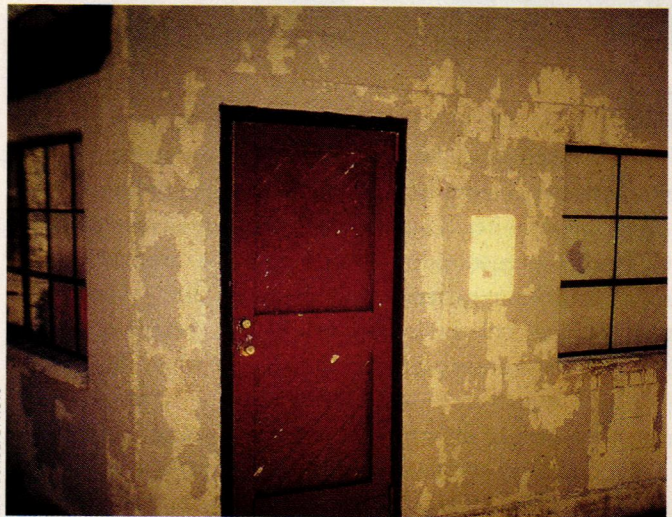
THIS PAGE: A circa 1790 house (top) in the tiny village of Niskayuna, New York, shows a restoration handled properly. Too often, poor prep or cheap paint can result in complete paint failure—like the above example on a building painted just six years ago. OPPOSITE: Repairs gone wrong can result in rot, failures, and cracks.
