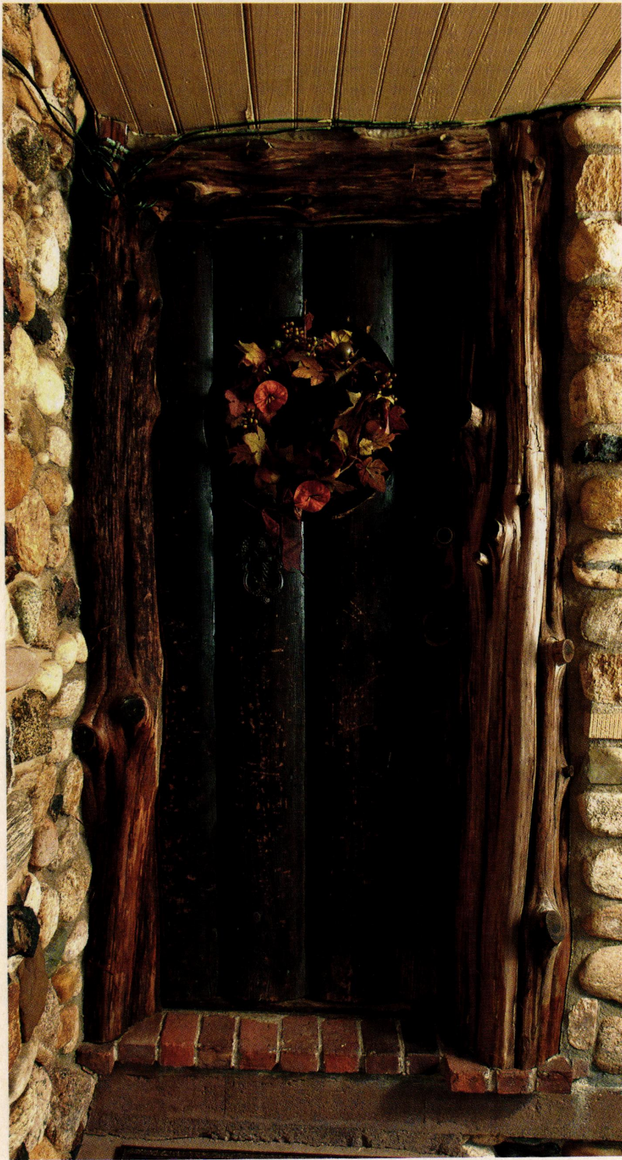
ABOVE: The house's solid, impressive log front door began life on a clipper ship, and has a cutout portal window (here partially hidden by a wreath). The Tortorellis had to get creative in their efforts to restore and weatherize the door.
