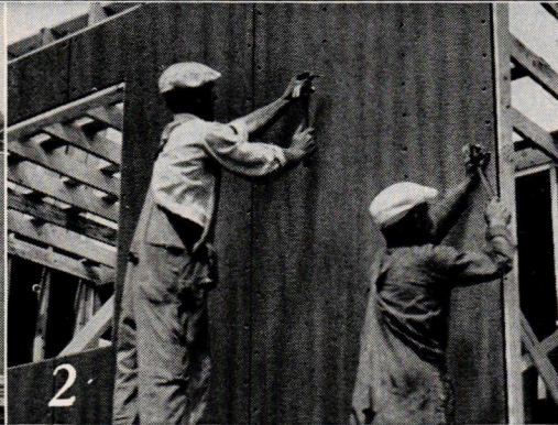
2 Applied quickly—every joint goes over stud, sill or header, thus reducing wind infiltration.
