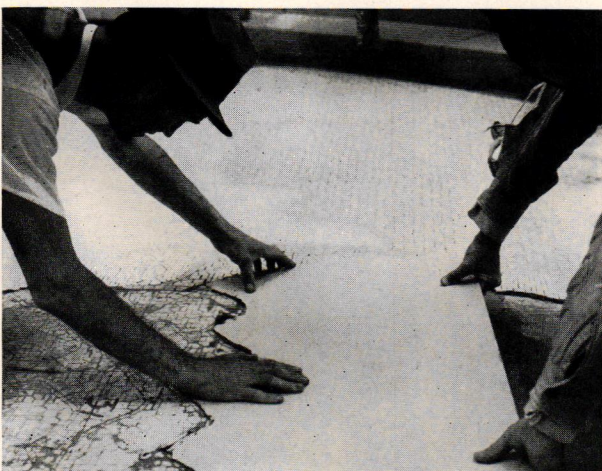
The tile sections are supported and stiffened by templates of wallboard, the same size as the numbered panels
