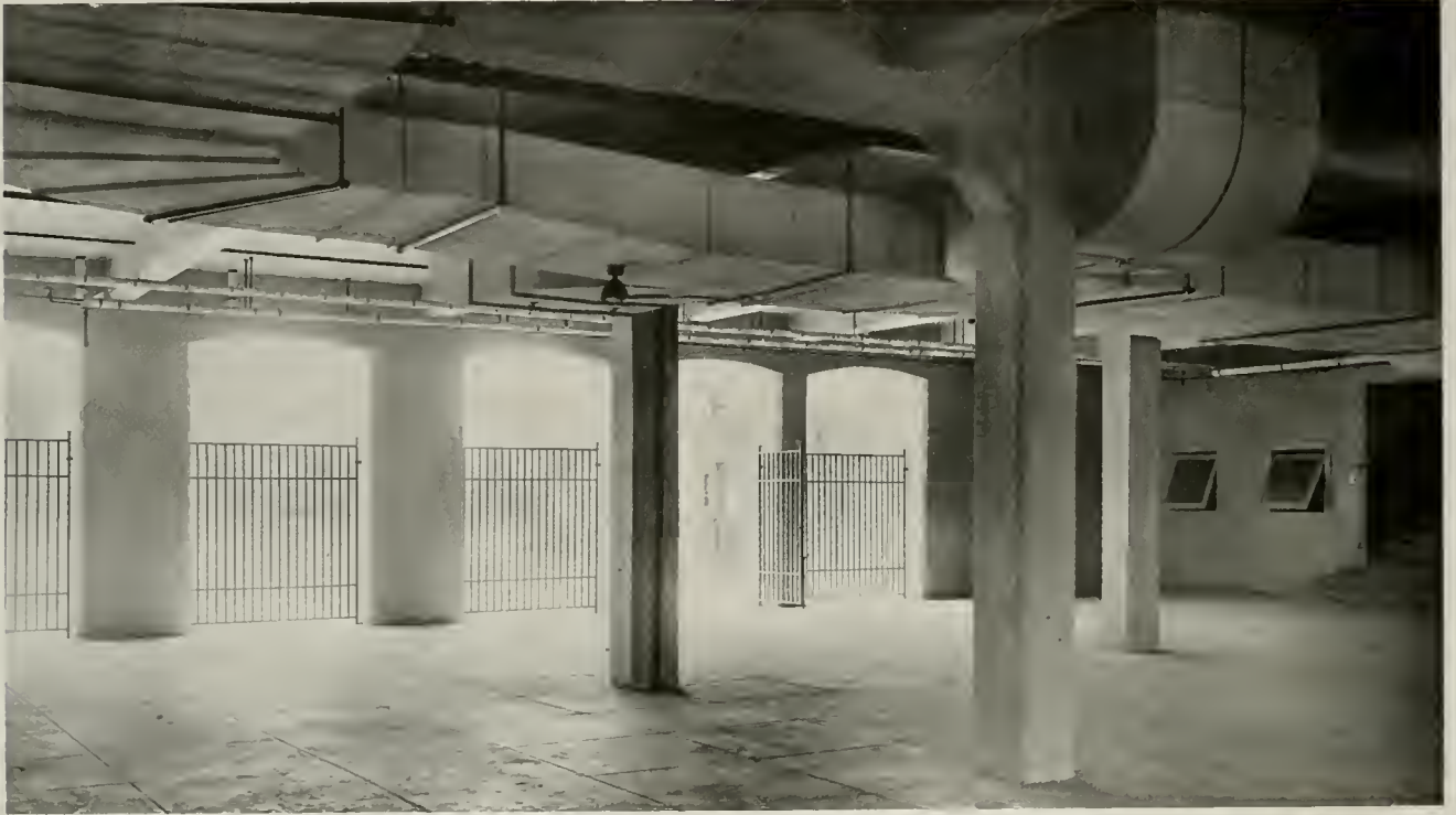
ONE OF THE GROUND FLOOR PLAY ROOMS, CLAWSON ELEMENTARY SCHOOL, OAKLAND, CALIF.
