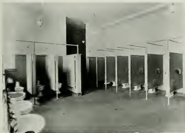
Typical Girls' Toilet Room, Benjamin Franklin High School, Portland, Ore. F. A. NARAMORE, Architect
