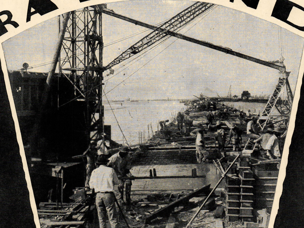
Laying the deck of the New Orleans Pontchartrain Bridge across Lake Pontchartrain, La. This bridge is supported by 2,796 reinforced precast concrete piles
