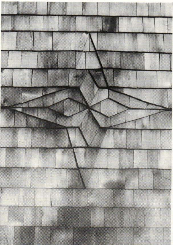
Example of the shingle installer's art created in heavy-butt Western Red Cedar by Liberty Cedar Co.
