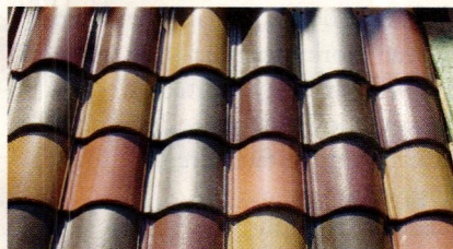
When replacing the terra-cotta roof of the Breakers mansion in Newport, RI, Boston Valley Terra Cotta used 35,000 field tile and approximately 4,000 special-shaped fittings.
