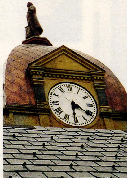
NIKO replaced the slate roof and sheathed the clock-tower dome in copper on the Hancock County Courthouse in Findlay, OH.
