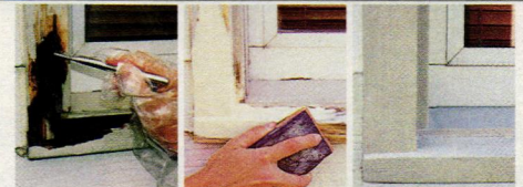
Restoration of rotted window is easy and cost-effective.
