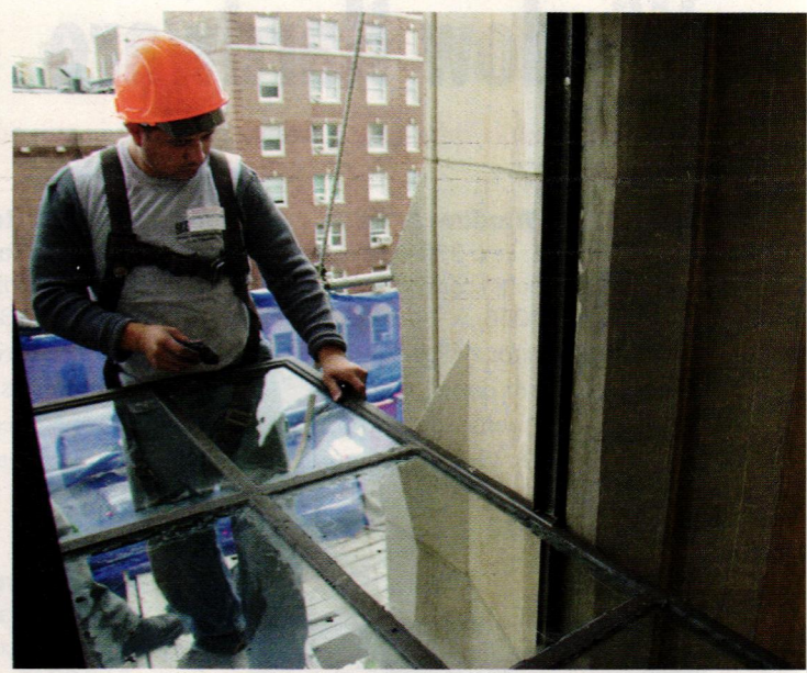
After the Columbia windows were restored in the shop, they were put back in the building where workers installed and putty-glazed the glass. Seekircher worker Omar Hernandez is shown here glazing one of the windows.
