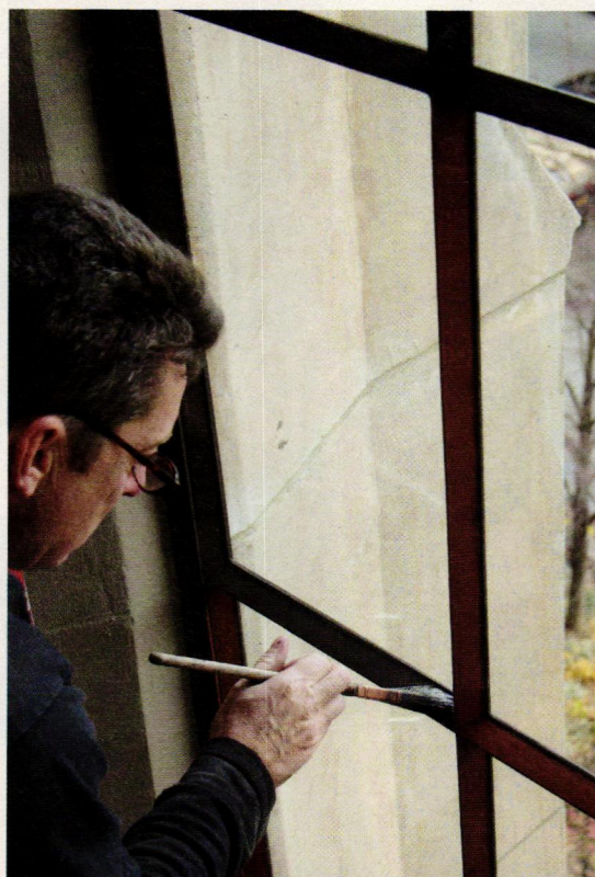
The final step at the Columbia University Hospital project in New York City was painting the windows. Ralph Whitehead of Seekircher applies two coats of paint.
