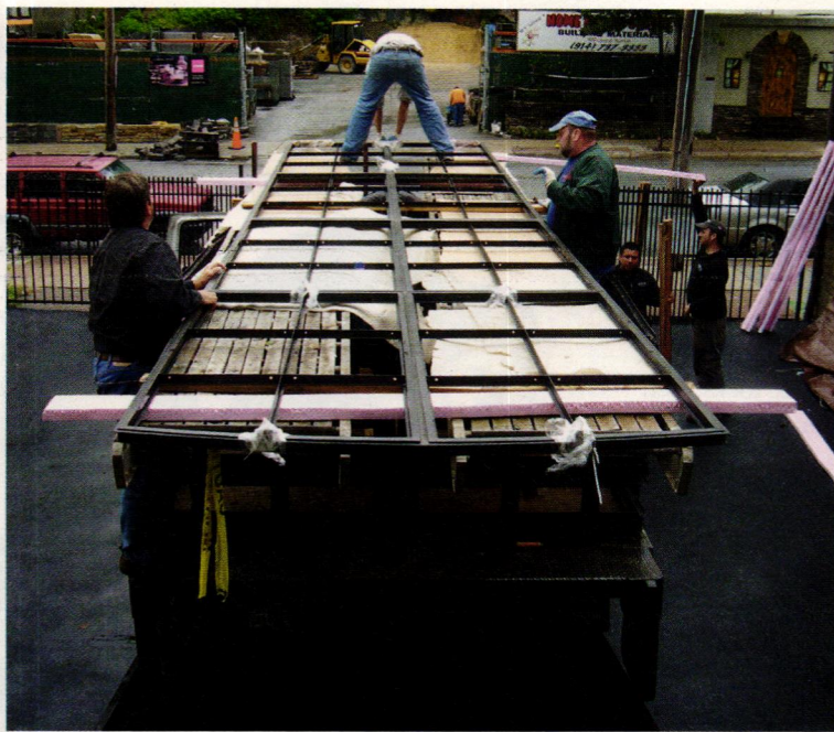
At Columbia University Hospital, the windows were taken out, loaded on to trucks and taken to Seekircher's shop in Peekskill, NY.
