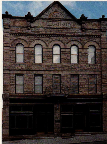
Allegheny Restoration completely restored and renovated the millwork, windows and entrance of the Dering Building in the historic city of Morgantown, WV.
