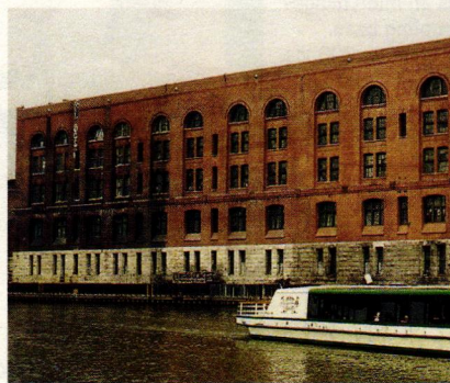
This building on the Milwaukee River has been partially cleaned with 101 Masonry Restorer from Diedrich Technologies.
