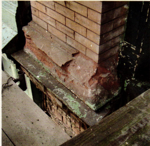
Before restoration, brownstone trim was falling away in chunks.
