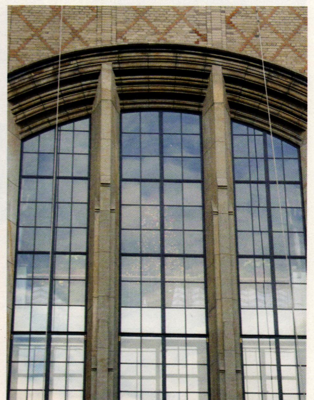
The restored steel windows at Columbia University Hospital now greet visitors as they enter the medical complex. Many viewers thought they were new. Photo: Richard MacDowell, Grenadier Corp.
