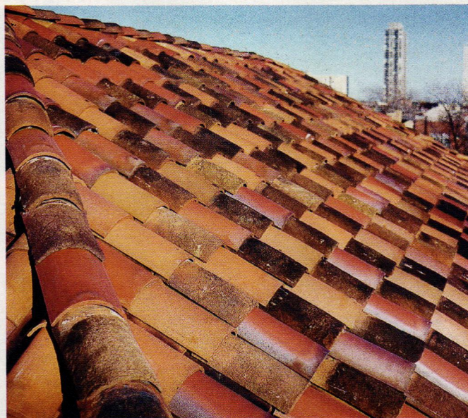
TOP: Tile Roofs supplied the salvaged red French tile and custom-made fittings for this old train depot in Fithian, IL. Photos (both): Tile Roofs, Inc.
