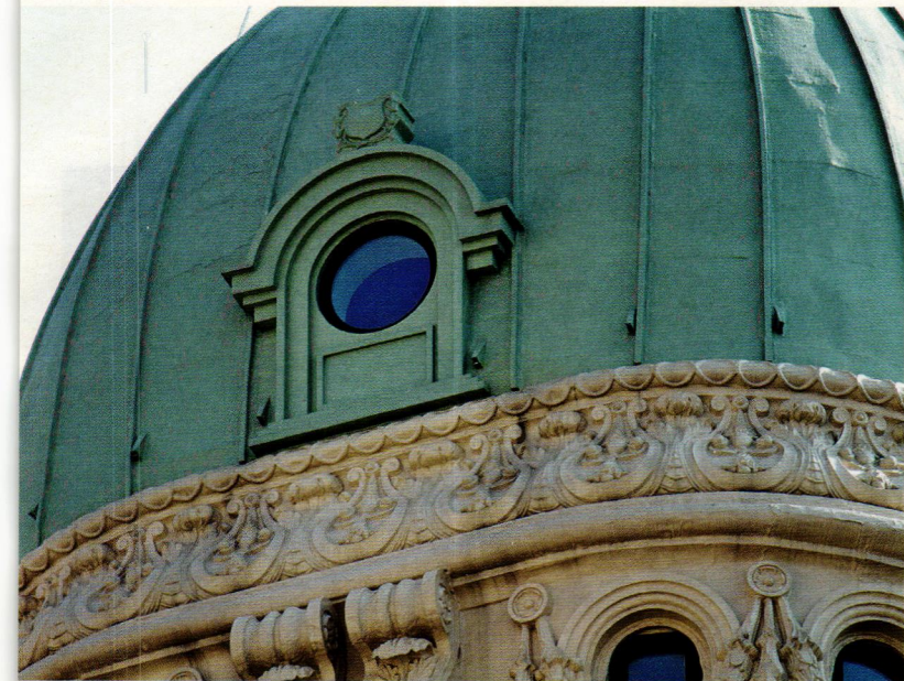
Gotham Metalworks fabricated this precision plasma-cut replication domed roof for a NYC landmarked building.
