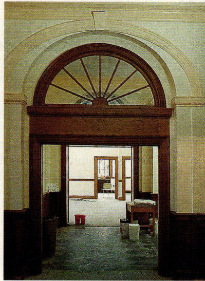
Architectural Components built the custom lunette, door frames, casing, chair rail and wainscoting to match the existing elements of this building.
