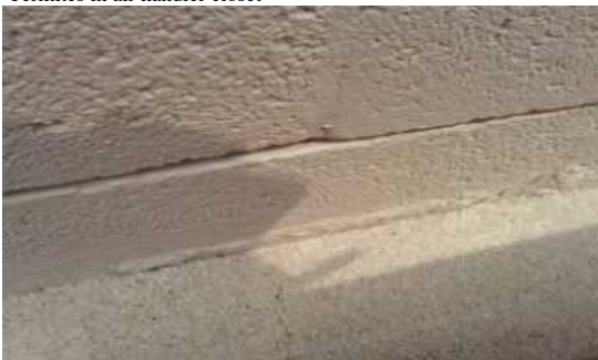
Water damage along walls
