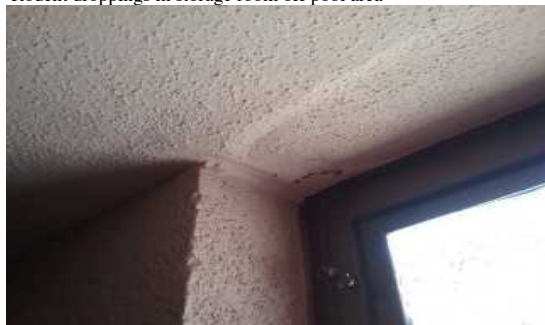
Water damage on ceiling in den
