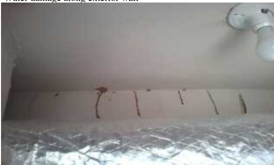
Termites in air handler closet
