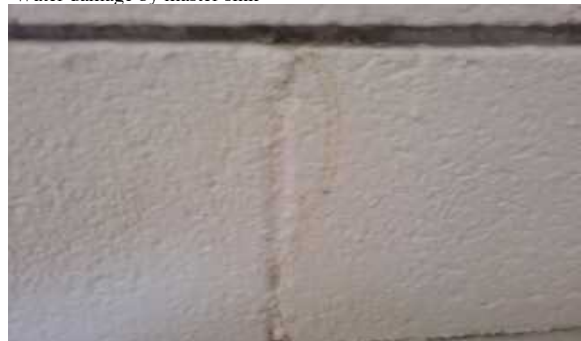
Termites on east wall in living room
