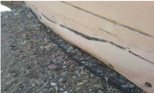
Water damage along exterior wall
