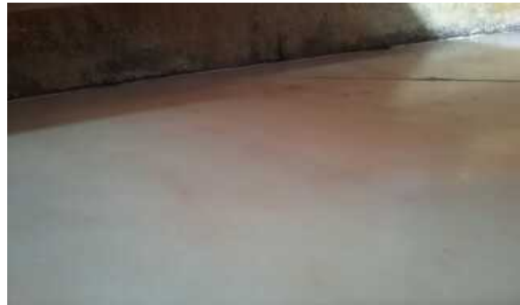
Water damage by master sink
