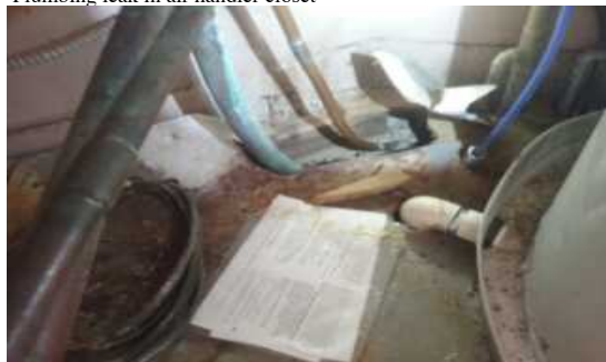
Rodent droppings in storage room off pool area
