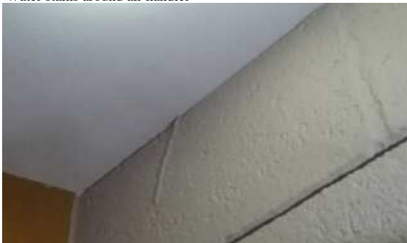
Termites in ceiling in guest bedroom with couch
