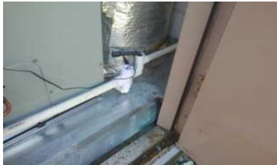
Plumbing leak in air handler closet
