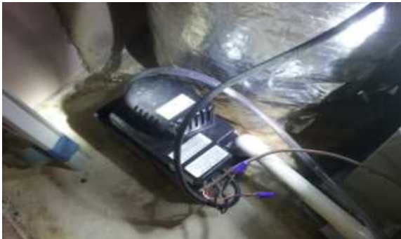
Water stains around air handler
